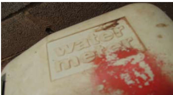
A pre-paid water meter.
